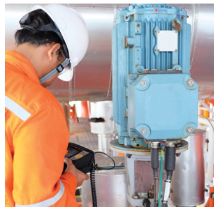
FIGURE 2. Vibration analysis uses data on the vibration signature along three axes
